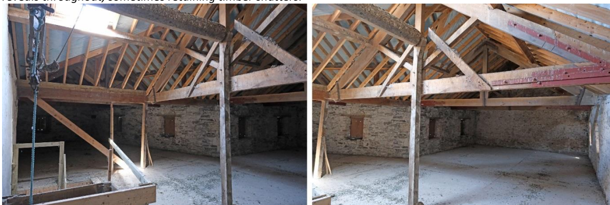
Fig.30: General view of the interior showing floor covering, plain walls and window reveals, and floor joists supported by structural timbers with steel bracing and timber columns.
