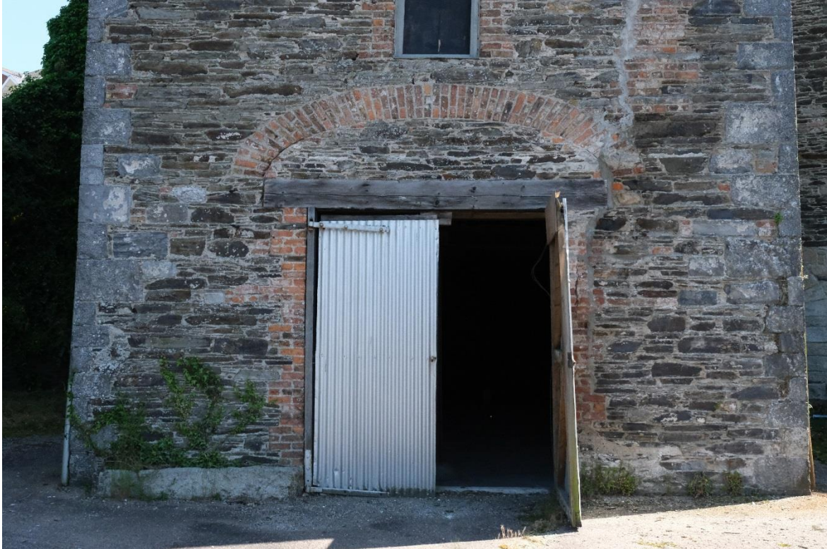
Fig.22: The courtyard level door of the return has a massive timber lintel and rubble masonry infill beneath a brick arch, with brick quoins. The elevation has limestone quoins (see Fig.14 also) and past repairs.
