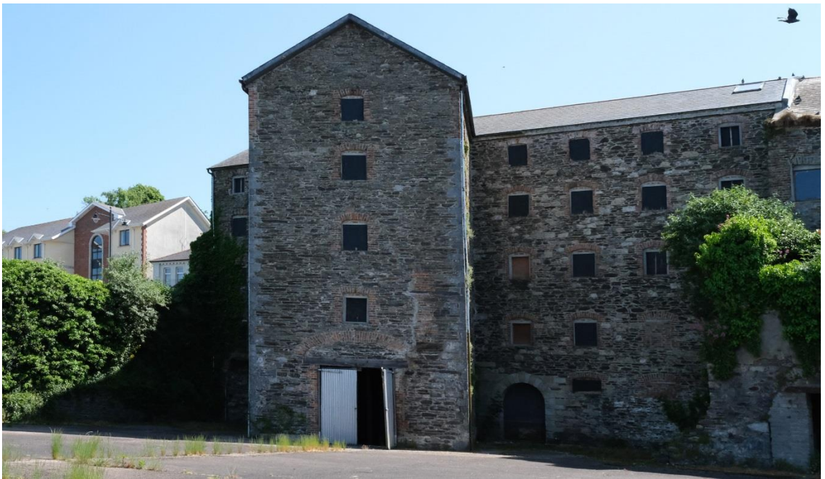
Fig.18: General view of the five-storey rear elevation (three floors at John Street level, and two basement levels) composed of random rubble masonry walls punctuated by camber- and segmental-headed brick windows, with granite used for the quoins of the return and for the arched doorway. The elevation shows a number of small repairs and alterations, but is largely unchanged from its appearance at the beginning of the twentieth century (compare Figs.10 & 11).
