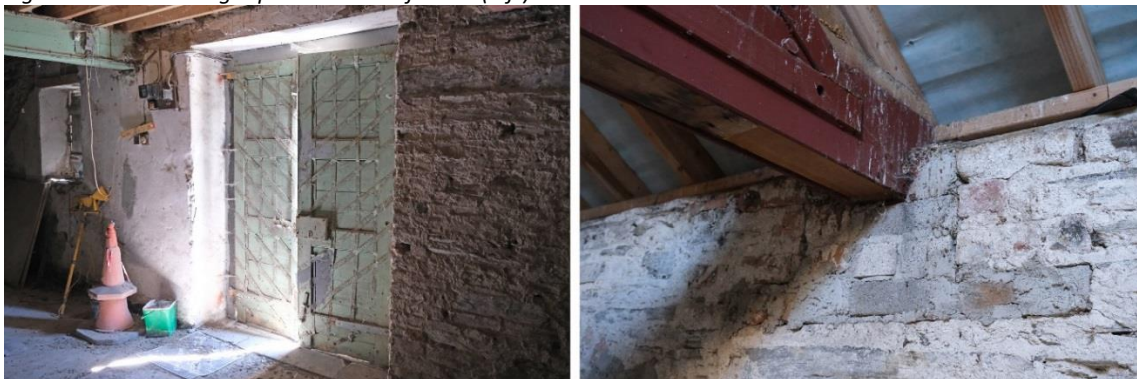
Fig.27: John Street level interior showing the southern doorway (left) which is a plain panelled timber door. The roof has been replaced, including replacement of roof timbers and the addition of bracing to existing timbers (right).
