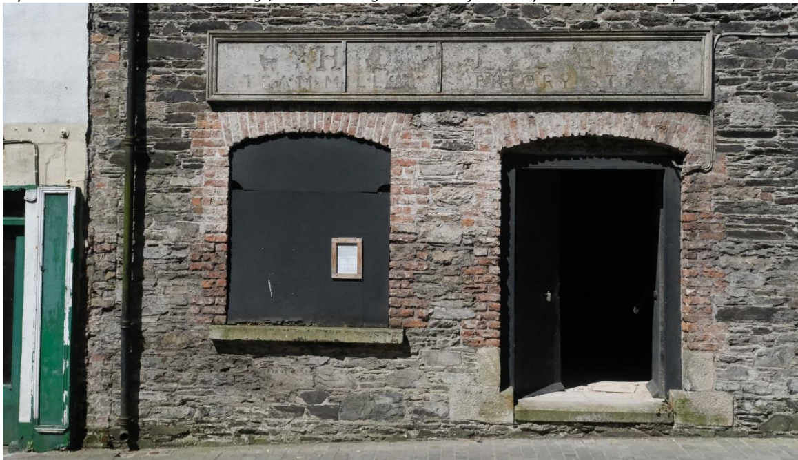
Fig.15: Ground floor window and doorway at the south end of the façade with signage plate above.
