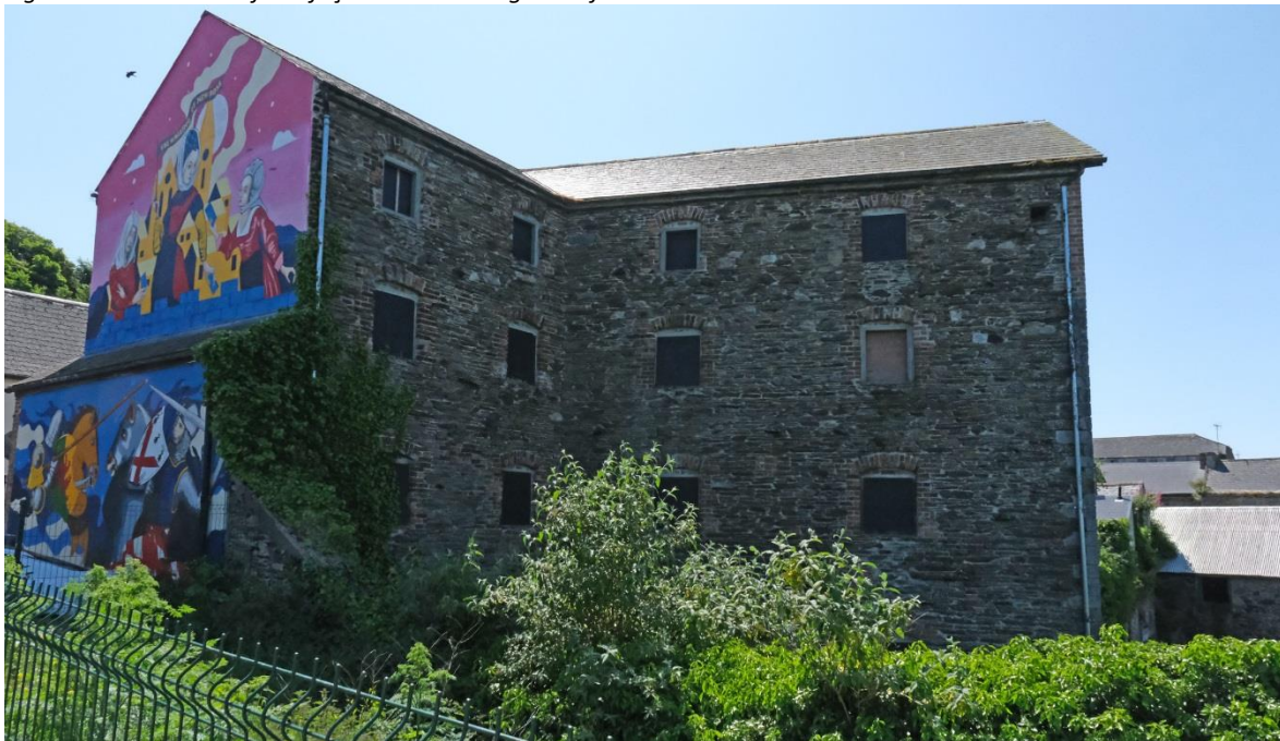
Fig.13: North elevation showing off-set return, mural on the north gable and slated roof and rainwater goods.
