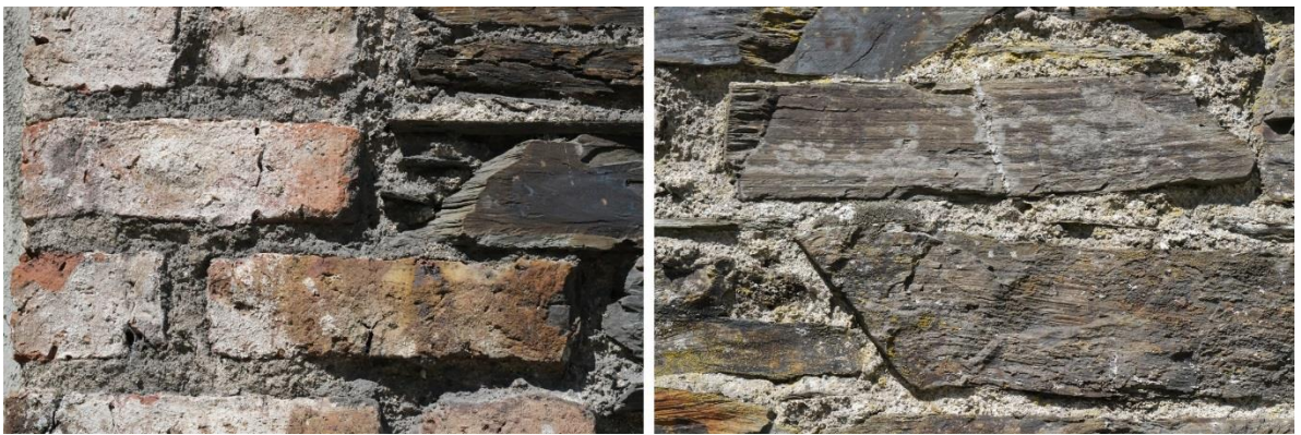
Fig.17: Detail of hand-made clamp-fired brick used to form door and window openings (left) and a detail of the locally obtained rubble stone used for the bulk of the masonry fabric (right) all bedded in a lime-based mortar.
