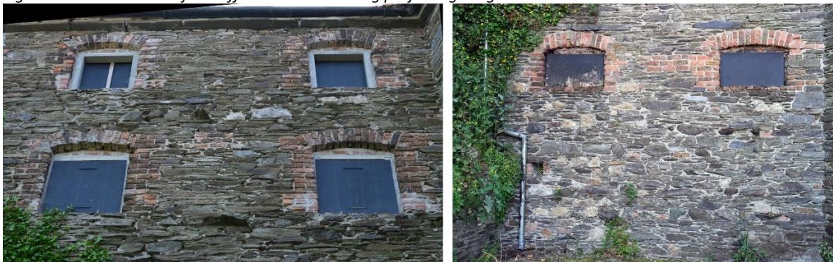
Fig.21: Details of the northern end of the west elevation showing the overhanging eaves course supporting the cast iron rainwater goods, brick window surrounds, and projecting rough corbels from the random rubble masonry walls.
