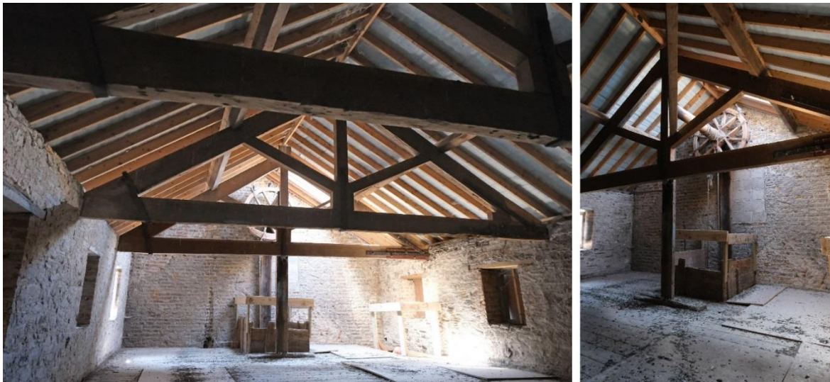
Fig.25: Top floor showing bare rubble masonry walls, roof timbers, and timber floorboards. Note blocked-up south window to rear of the winch. The window reveals have timber lintels, and some internal timber shutters survive.
